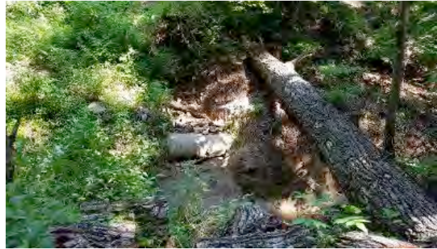
Exposed water main and downed tree in Tributary B
